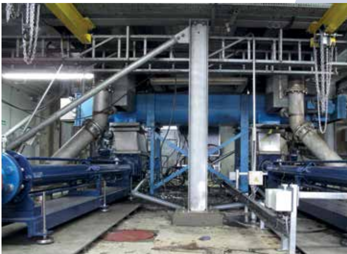
SEEPEX pumps installed at Reading STW
