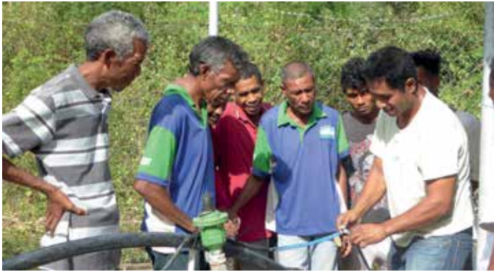
Figure 1: BESIK pump technician Luis Fernandes installing a new pump at Romoco in Lautem District.
