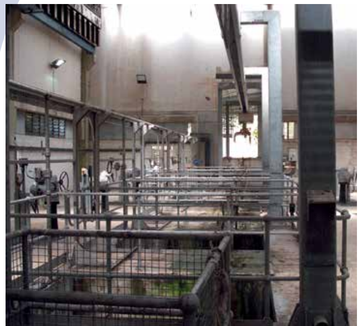
The Bosker installation at Thames Water's Deephams WWT works serves several inlets
