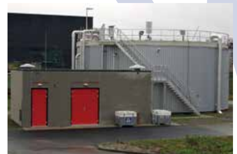
Figure 4 – The DEMON® installation at Amersfoort, NL has been operational since 2012 (Image courtesy of Sweco)
