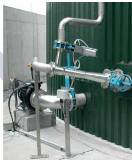
Landia's externally mounted GasMix AD digester mixing at Tullamore WWTW
