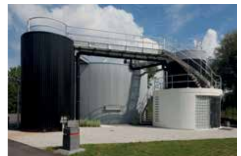
Figure 5 – The DEMON® installation at Nieuwegein, NL has a capacity of 450 kg/d (Image courtesy of Sweco)
