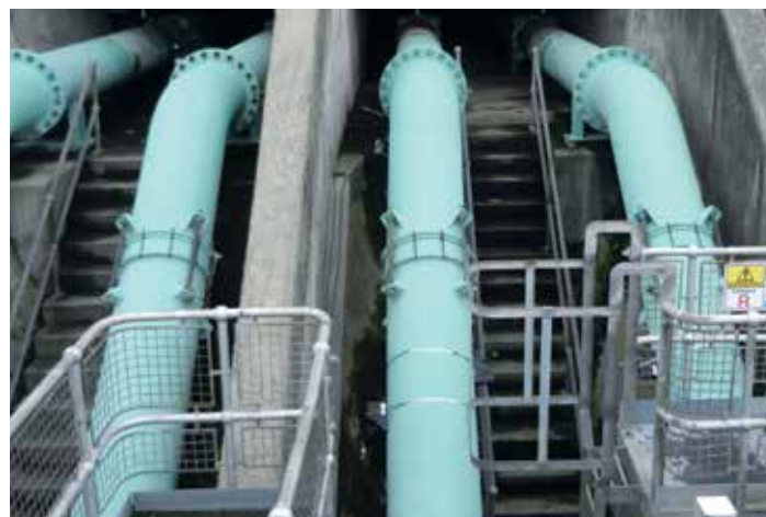
Sewage pumping stations receive raw sewage from underground pipelines and continually lift it to higher elevations until it reaches the designated treatment works.
