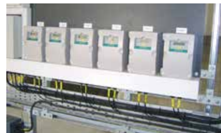
Sitran FST020 clamp-on ultrasonic flowmeters have made it possible to monitor each sewage pumping station remotely, eliminating the need to send operators out into the field and allowing operational staff to be deployed more effectively.
