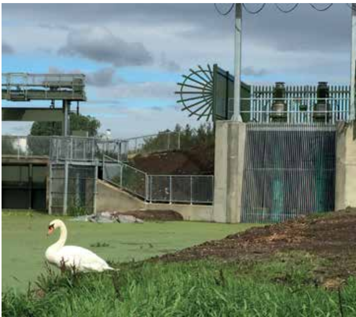
Webb's Hole Pumping Station
